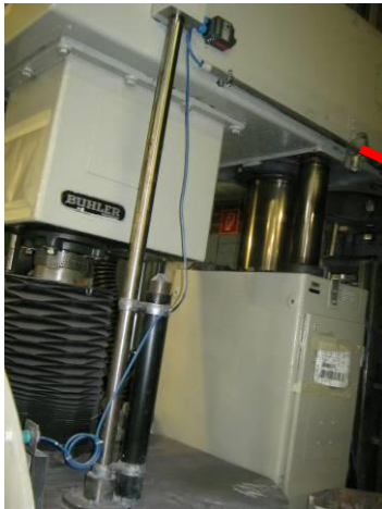
Picture 8 (Low position switch)
